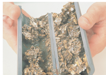
Figure 11-CS11_01 Zebra mussels clog pipes.
